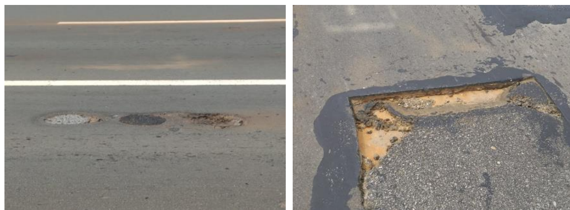
(a) 坑槽、修补二次破坏、开裂、返锈
