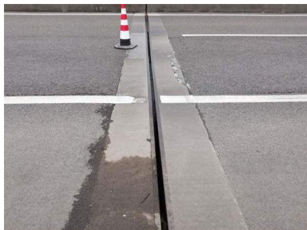
锚固区砼破损
