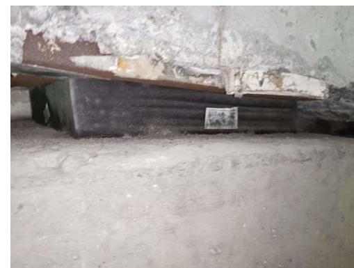
图2.2-91 左幅8-7-1#支座剪切变形
