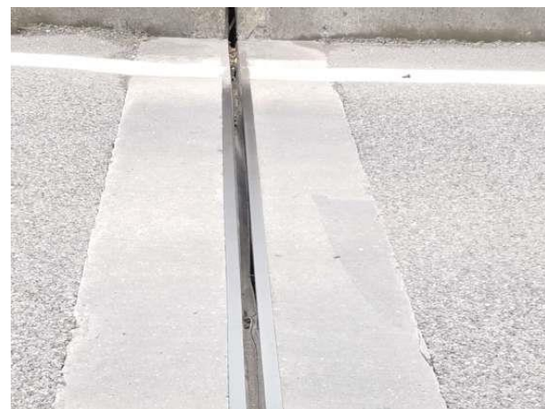
锚固区砼破损
